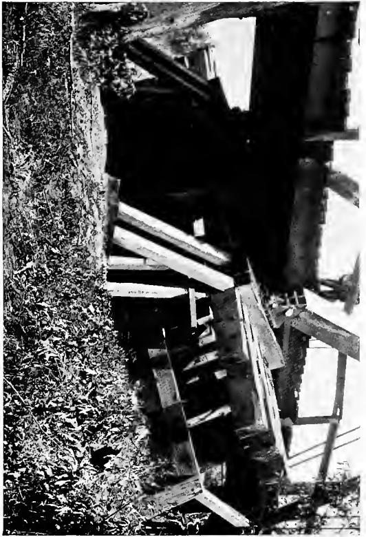
A. Bridge over Salinas River, 4 miles south of Salinas. South terminal pier thrust south 7 feet. A. C. L.
